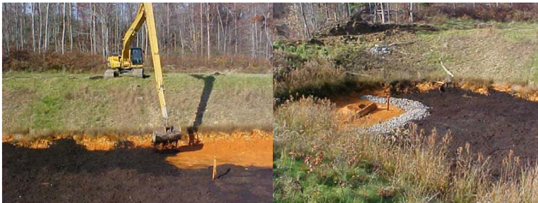
Figure 6. Distribution of new compost (left) and placement of rocks to hold compost in place near the distribution pipe (right).
