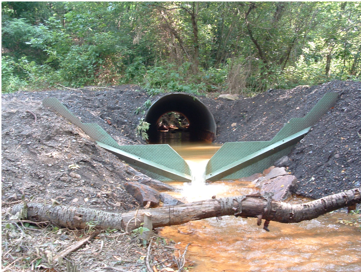
Scarlift Site 36 – 0 (usually) to 2 mgd flow Double V-notch weir for flowrate measurement
